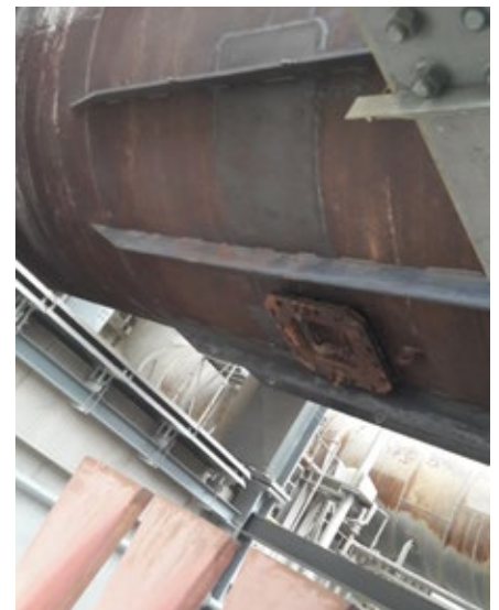
Kiln crack repair
